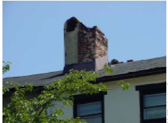
Example of chimney deterioration
