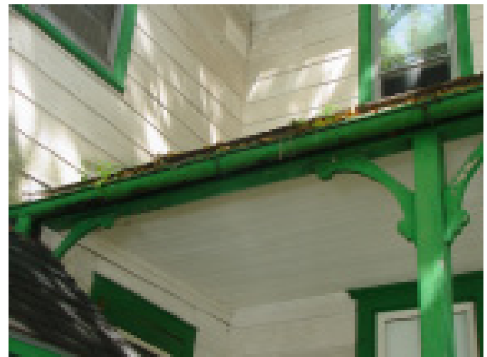
Gutters full of leaves and debris
